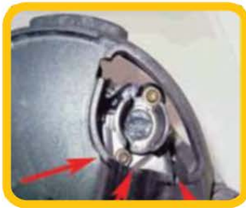
Discolored/Burnt Terminals Terminal not tightened correctly
